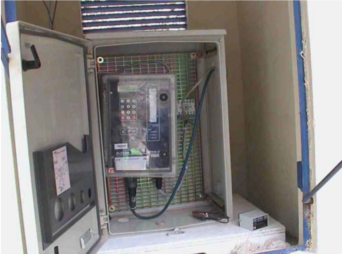
Figure C.18: EPROM Datalogger installed at Lake Artesoncocha (4200 m a.s.l.) where runoff is recorded. Photo taken by Bernard Pouyaud.
