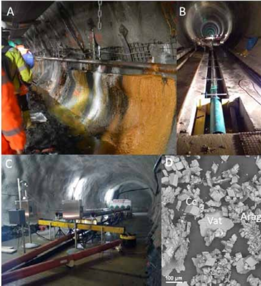
Figure 1. Diverse mineral precipitates (A) in the course of continuous groundwater discharge underground can block a tunnel drainage system (B) and were investigated by in-situ field tests (C) targeting an increased process understanding of the precipitation conditions (e.g. D: CaCO 3 polymorphism) as well as efficient countermeasures (e.g. optimized drainage design, addition of inhibitors).
